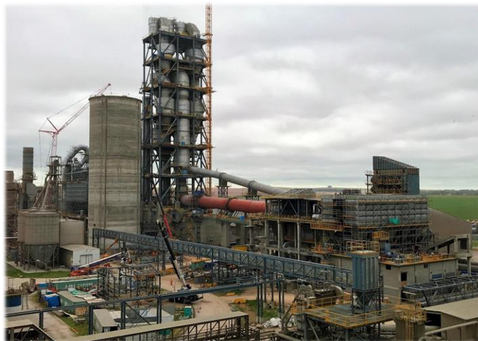
L'Amalí2: Mill, Preheaters, and Kiln
