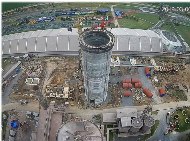
L'Amalí2: Mill, Preheaters, and Kiln
