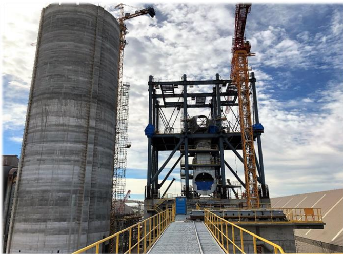
L'Amalí2: Silo, Preheaters, and Kiln
